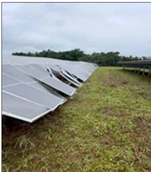
Figure 3. Panels after floods.
